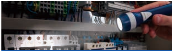
Erroneous circuit-breaker activation
